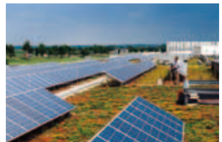
6. Roof with fully-installed solar energy system.
