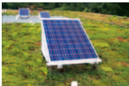
The test involved two modules installed on a “naked” membrane panels being compared with one module installed on a green roof. In each case, attention was focused on the temperature at the underside of the panels.
